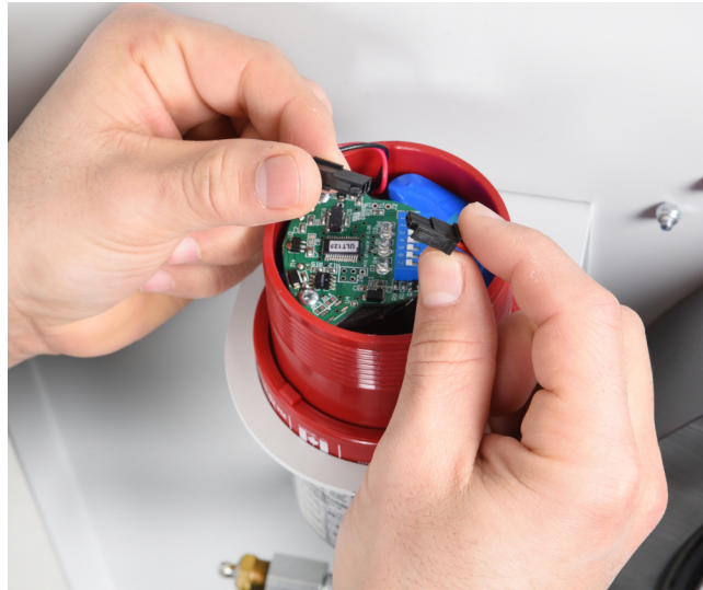
Figure 78. Plugging the battery pack to the connector inside the lubricator's unit.
