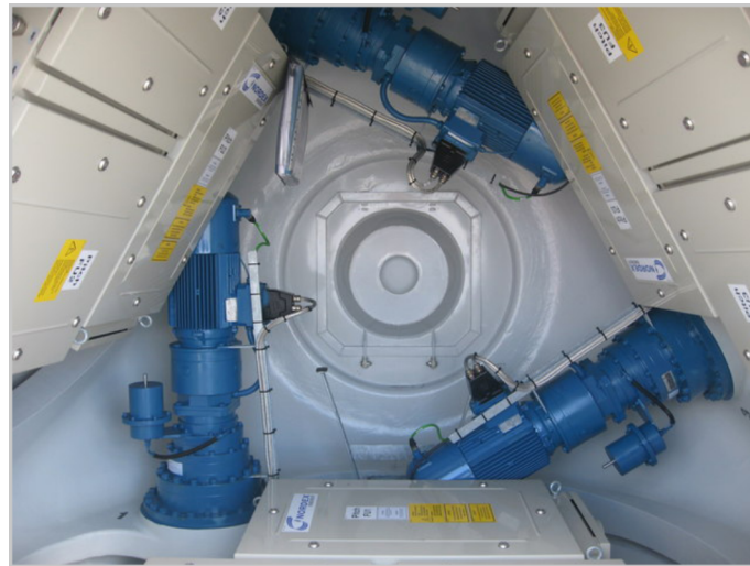
Figure 56. Electrical pitch system using servomotors.
